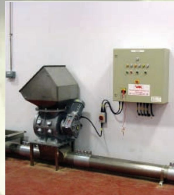
MLD 400 in use at Exotic Farm Produce
